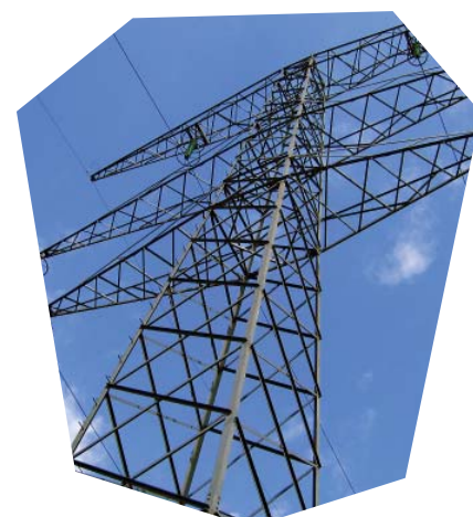
High-voltage power line
