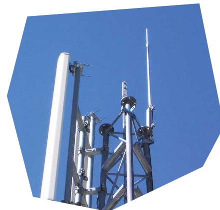
Mobile telephone antenna
